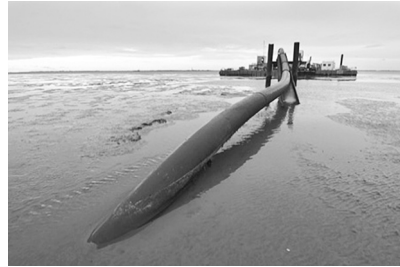
from The German Offshore Wind Energy Foundation Figure 7 The Cable Route of Offshore Wind Power in the North Sea
